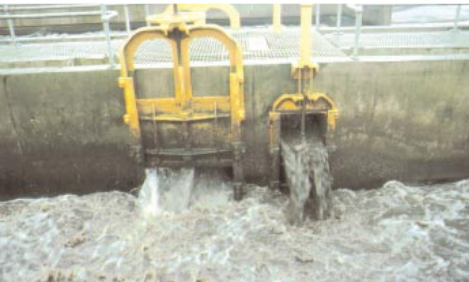
LEFT: Part of an activated sludge aeration tank from a sewage treatment works showing inflows of settled sewage (lighter coloured inflow) and re-circulated sludge (darker coloured inflow). Once again this is a likely source of many uncultured bacteria known only from their 16S rRNA gene sequences.
